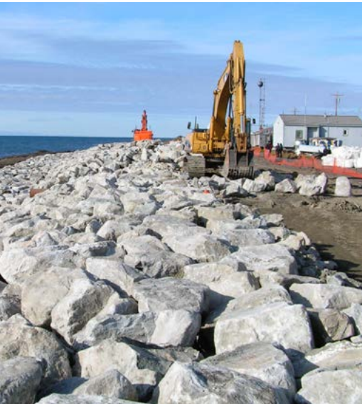
Rock revetment in Kivalina, Alaska. Image credit: John Farrell, USARC
